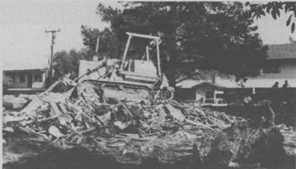
A bulldozer, sitting on the pile of rubble January 12th which, until the previous week, had been a community house known for twenty years as "The Well."
